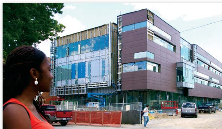
Construction of the new Medical Education Building at the University of Windsor gets a close look from Civil Engineering student Ogheneruemuse (Christy) Ekepekeude.
